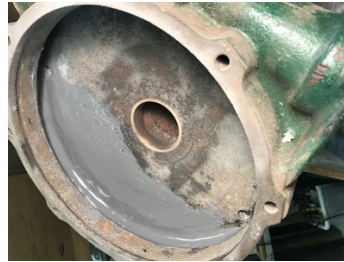
Inside of pump casing shows Belzona 1212 used to fill the crack and create a smooth finish for the water flow.
