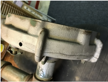
Depicts crack on pump casing.
