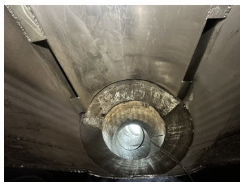
Chute after a thorough cleaning was performed.
