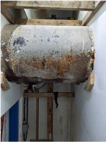
Defective pipe in need of reinforcement.
