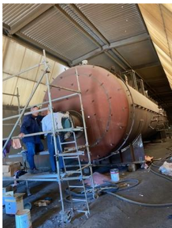
view of vessel
