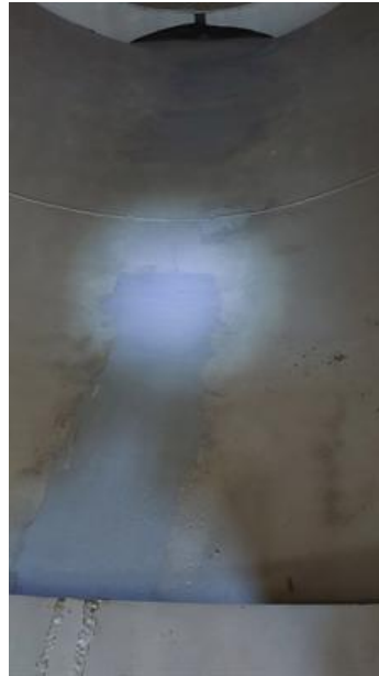
Fixed tank bottom
