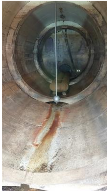
Damaged tank bottom
