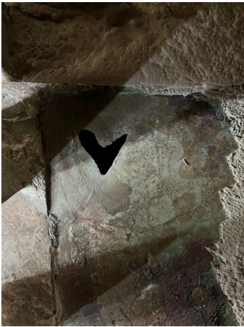
Internal through hole defect.
