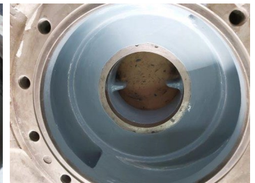
Once the surface was rebuilt, Belzona 1321 (Ceramic S-Metal) was applied to enhance protection and prevent further damage.
