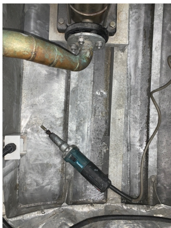
Engine room flooring to be repaired.
