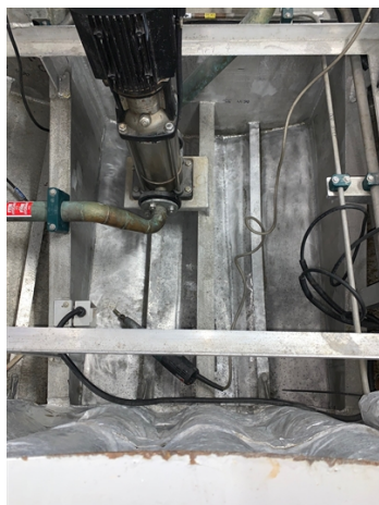
Surface preparation carried out using handheld power tools due to confined space.
