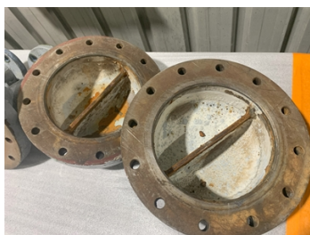
Existing condition of HVAC end covers suffered erosion & corrosion
