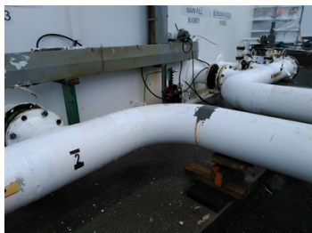
Pipeline to storage tank.
