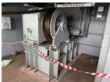
Winch housing in question
