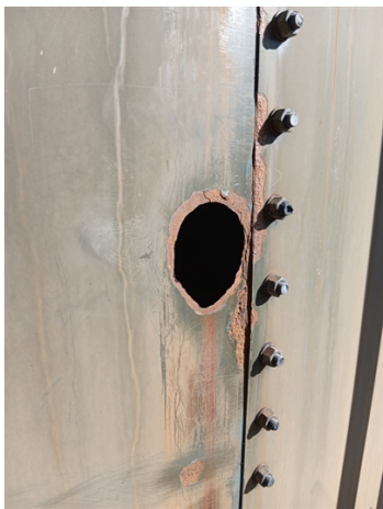
Through wall defects from internal chemical attack and environmental exposure
