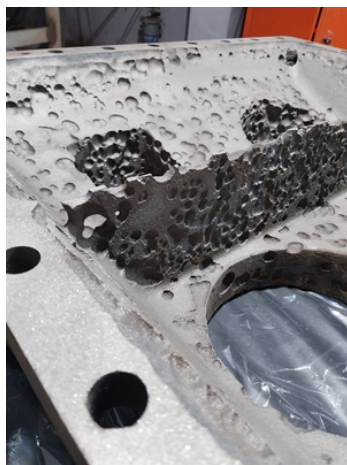
Severe metal losses
