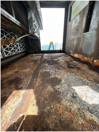
Air handler unit condition before Belzona treatment
