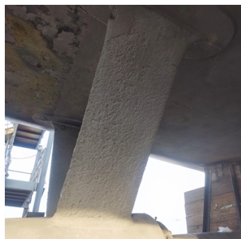
Corrosion attack was caused by prolonged exposure to seawater
