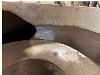
Belzona 1311 Ceramic R Metal applied internally to rebuild the hole at the cutwater
