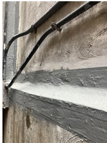
This is a close up on the 3121/9331 repair on the horizontal and vertical joints, after the job was completed.
