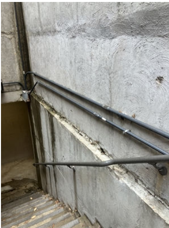
This image shows the leak externally in the vertical and horizontal joint of the wall.
