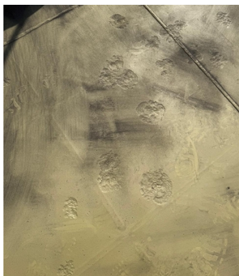
Multiple damaged locations on the steel deck
