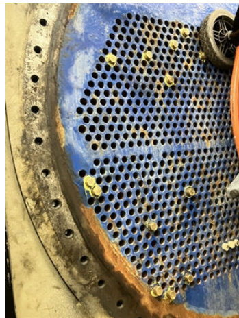
Close up image of the tube sheet showing failed enecon coating with creep corrosion around circumference.
