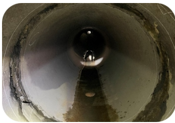
Damage on the flange of circulating water pipe discharge circulation pipe
