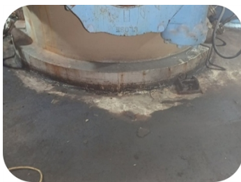
Damaged on the lower section of condenser waterbox
