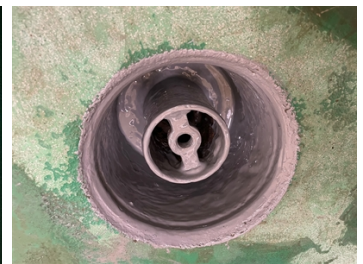
Condition of the scupper after 1 month in service
