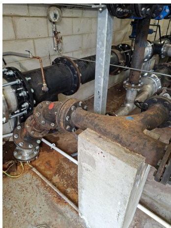
Pipework exhibiting surface corrosion due to ongoing condensation and moisture exposure
