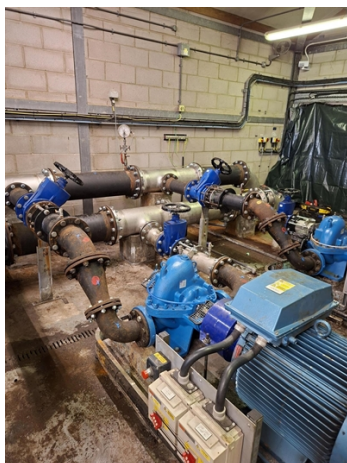
Degraded external surfaces showing clear signs of corrosion under challenging atmospheric conditions
