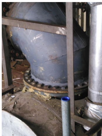
Leaks around flange
