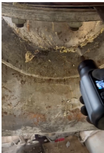
Close up of leaking areas
