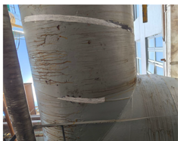
Leaking pipe with sand holes
