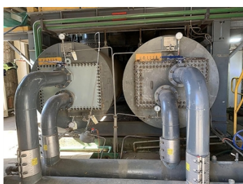
Nickel smelter intercoolers in need of repair
