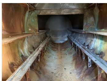
Significant corrosion of the main shell and internal components.
