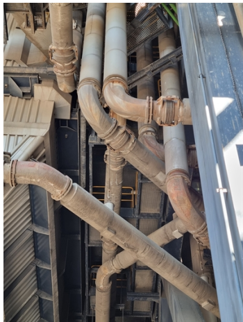
Pipework leading from the coal mill to the burners.
