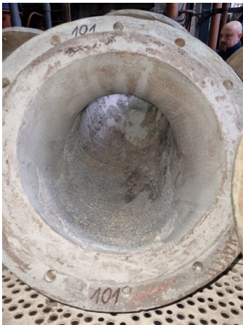
Pipe elbow showing remnants of the previous Belzona 1812 application.
