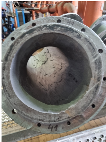
One of the most severely damaged pipe elbows before application.
