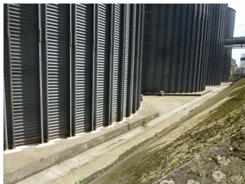
Tanks before the application
