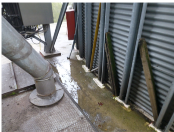
Condition of the problem areas
