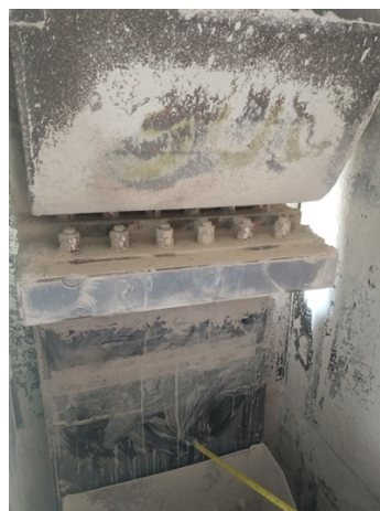
Front view of the bucket elevator belt showing the corresponding repair location.
