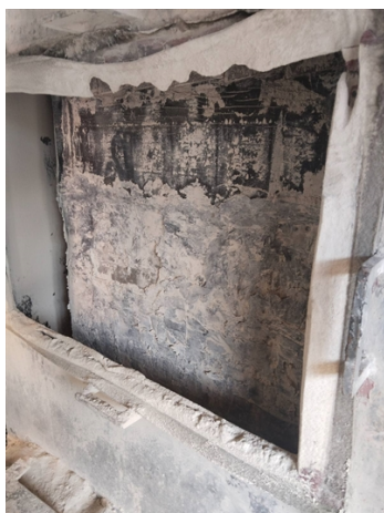
Close-up of the damaged bucket elevator belt showing severe rubber deterioration and material loss prior to repair.
