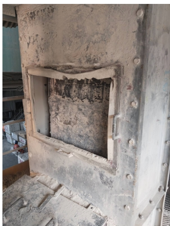
Rear side of the bucket elevator belt showing severe rubber damage prior to repair.
