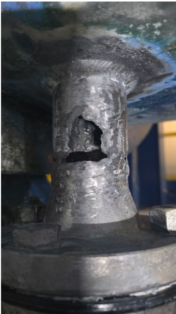
The damaged nozzle.
