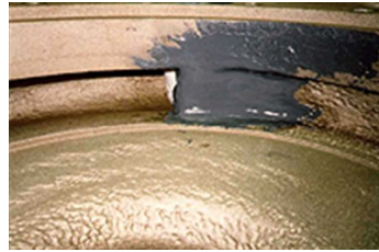
Rebuild of badly eroded cutwater using an Elastomer former to obtain correct profiles
