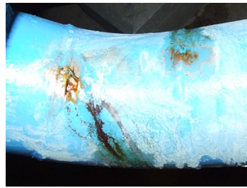
Close up of leak
