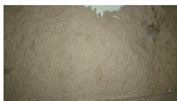
Corroded and damaged surface.
