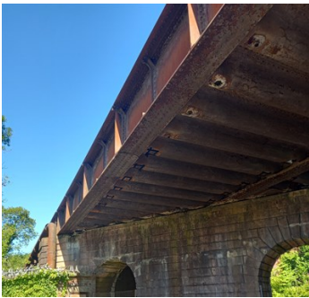
Bridge with leaking sections
