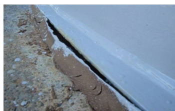
Original mastic failure
