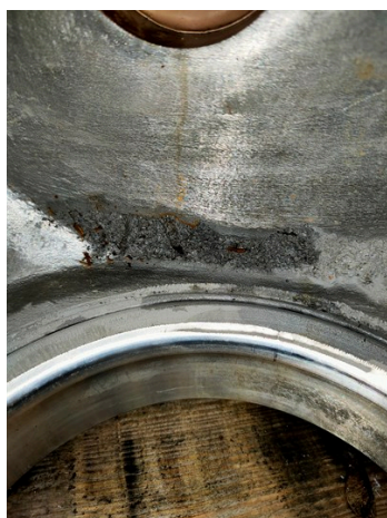
Close up of the cavitation damage
