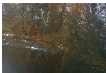
Initial state of the damage
