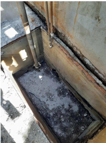
Damage to the sump pit area.
