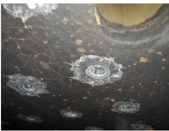
Cracking on the original rubber lining
