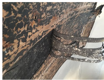
Delaminations on the original rubber lining
