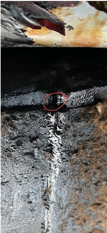
Pinhole leak in oil jacket
