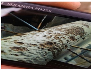
Pitting on pipe
