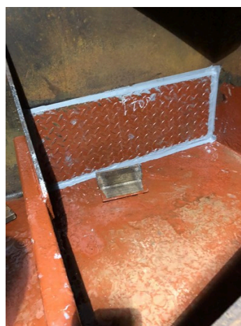
Plate applied to the corroded area
