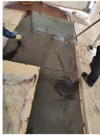
Utilisation of a roller between each layer to remove bubbles and consolidate.
