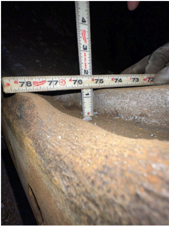
Showcasing and measuring the damage caused by the corrosion.
