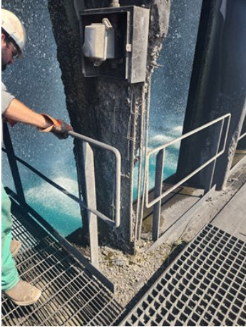
Deterioration of the columns
