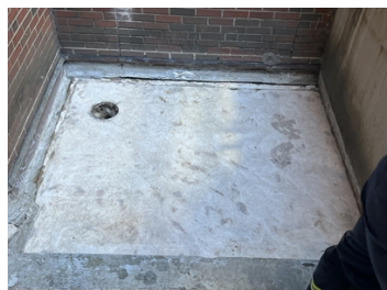
Old Coating was removed and floor was taken to bare concrete by a diamond grinder.
