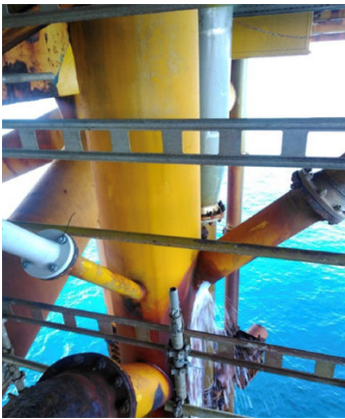
Severe corrosion on 24" caisson.
