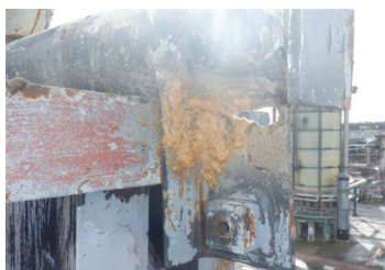
Corroded section covered in wax oil
