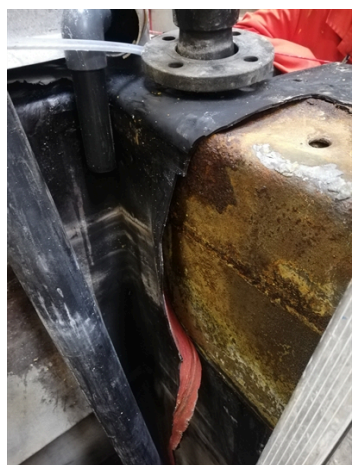
Ebonite tank suffering from degradation
