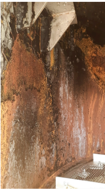
Traces of severe corrosion from under the rubber lining
